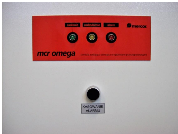
Fig. 3 Enclosure door – signal panel and reset button.
