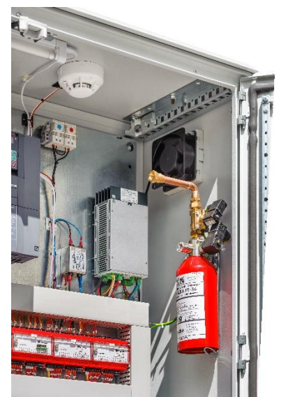
Fig. 13. FFES inside the panel.
